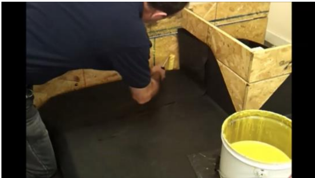
Fig 3: Applying the bonding adhesive to the back wall and the mating surface.
