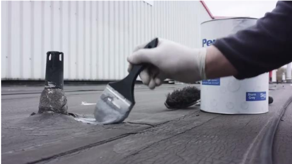
Fig 5 – Working the Emergency Roof Repair into the damaged area of the flat roof.
